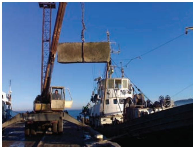
Fig. 3. Concrete mooring block for longlines (approximately 10m 3 or 23 t) destined for deployment at the IPA mussel farm at Gonio being loaded at the port of Batumi. Photo by Enrico Beridze.
